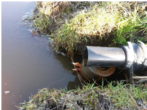
SorbiCell in de drain
